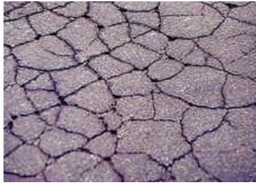
Figure 1. Late Stage Alligator Type Fatigue Cracks
